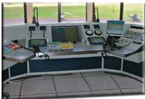
Fabricated New ATC Console
